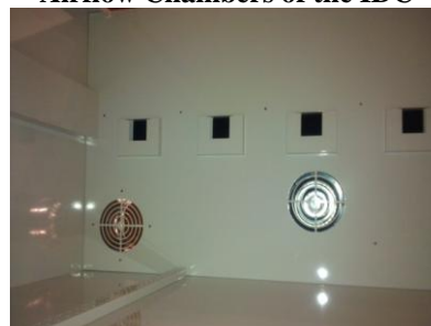
Airflow Chambers of the IDC
